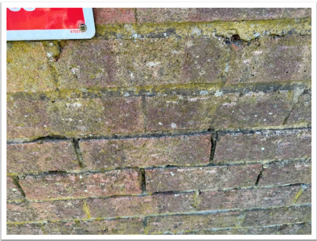
Photo 3: Localised brick spalling and weathering to external wall.
