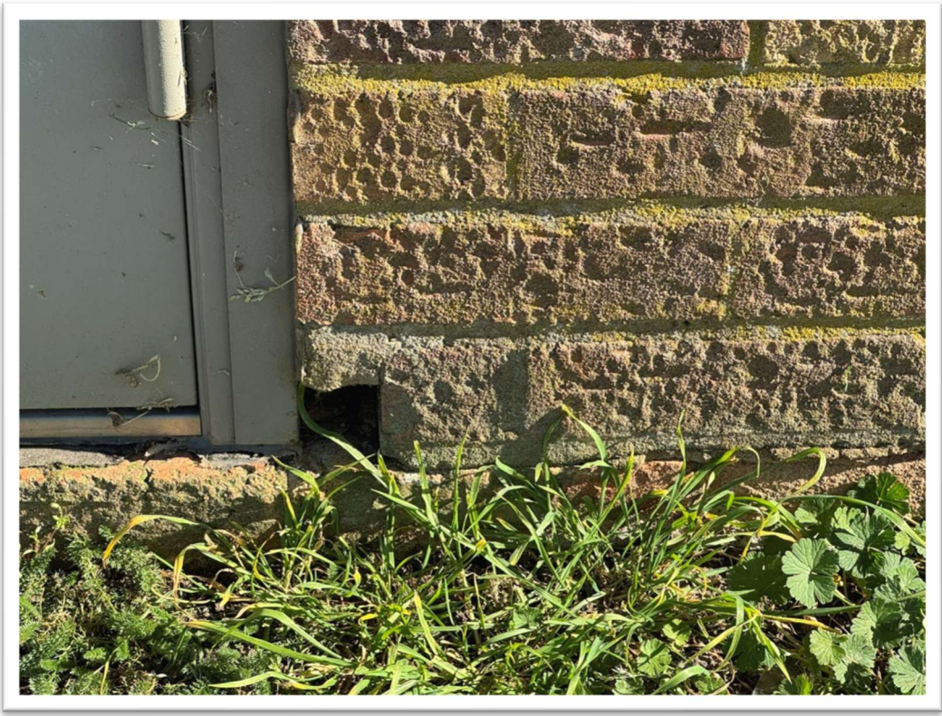
Photo 4: Localised missing brick at low level to external wall
