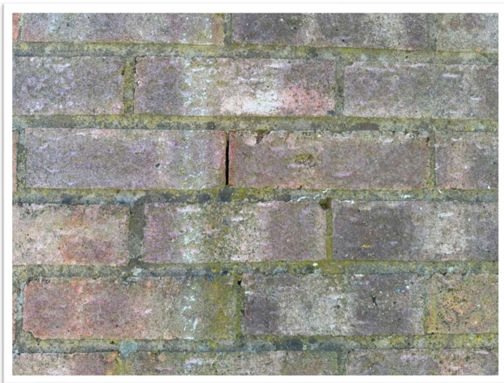
Photo 2: External brickwork with minor vertical cracking to mortar joint
