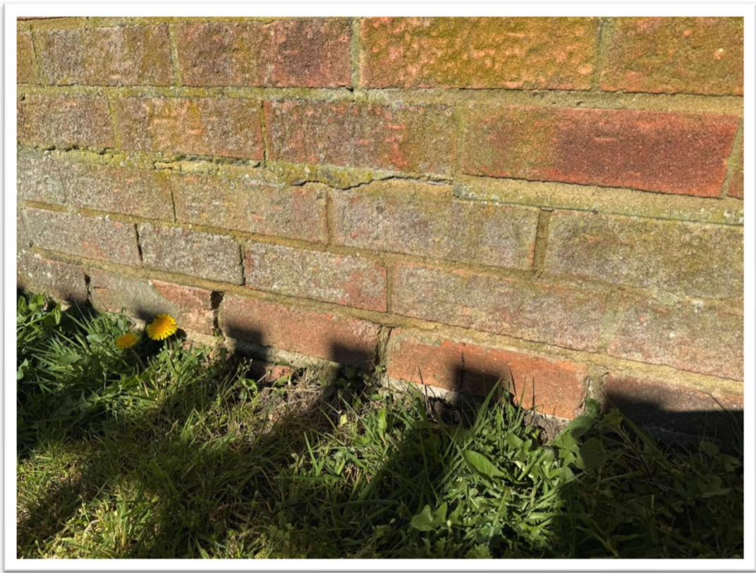
Photo 7: Horizontal cracking and mortar deterioration to external brickwork
