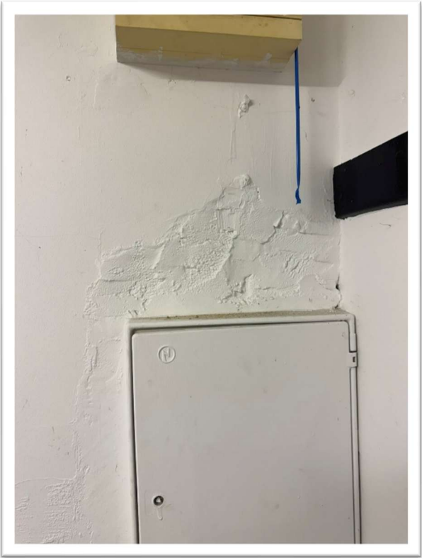
Photo 10: Internal wall with previous repair and uneven plaster finish
