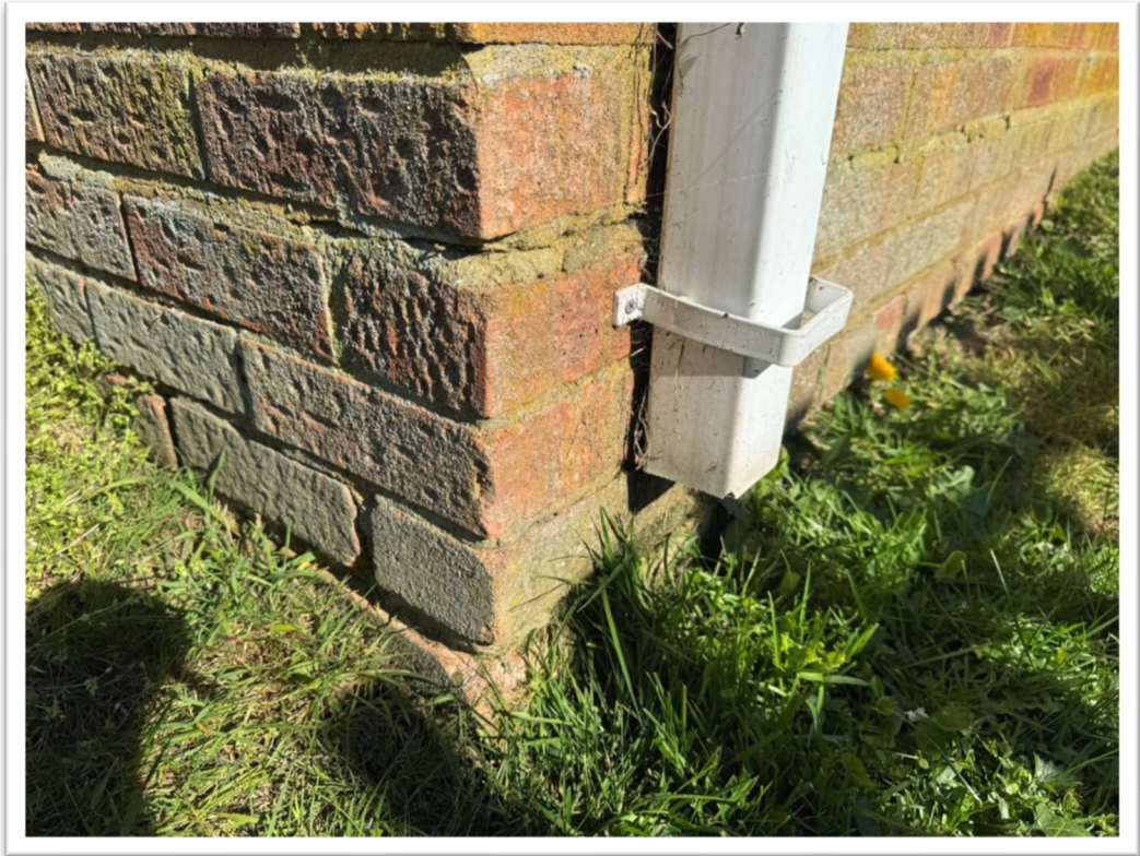
Photo 6: Downpipe discharge adjacent to wall with potential for water saturation
