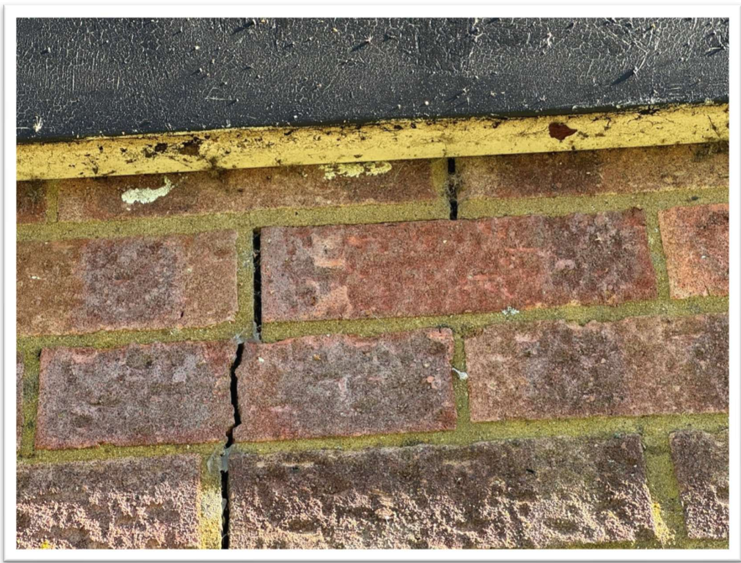
Photo 5: External wall above opening showing localised cracking
