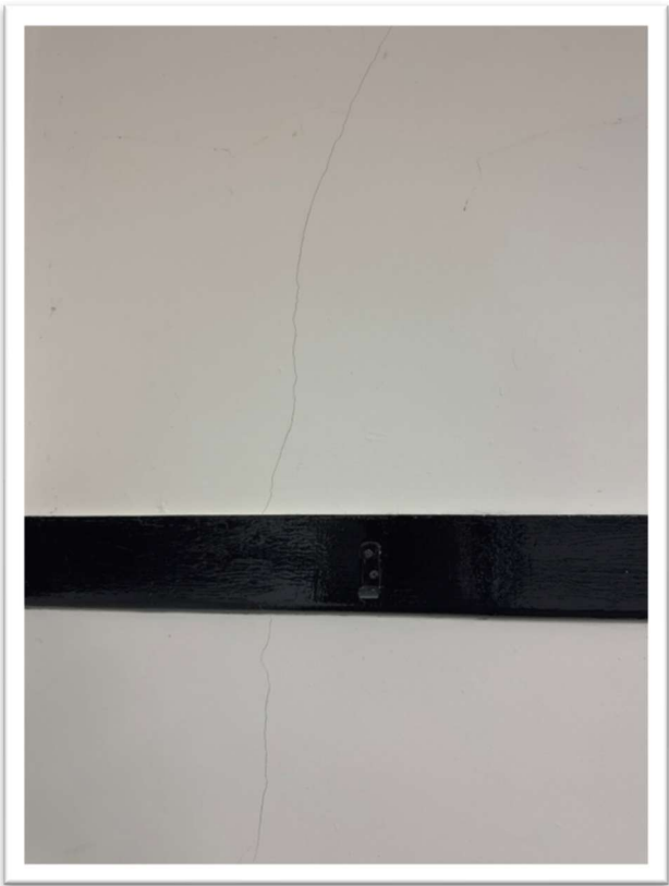
Photo 9: Internal wall with vertical hairline cracking to plaster finish
