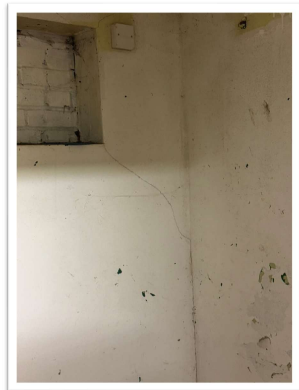
Photo 12: Internal corner cracking and localised surface deterioration
