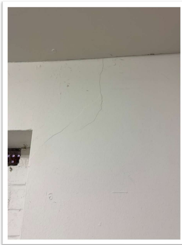
Photo 11: Internal cracking at wall/ceiling junction
